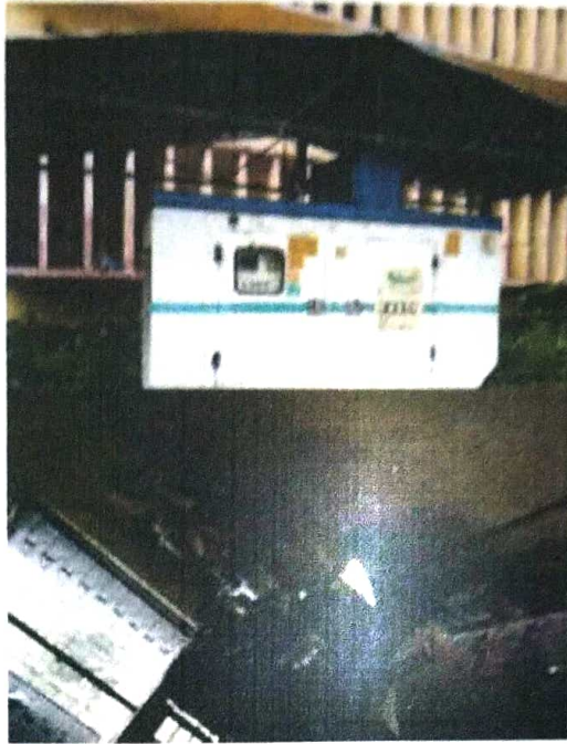
Two generator at our college
